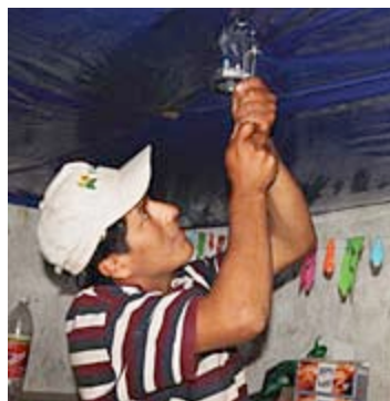
Each lamp is attached to the ceiling with screws and wired to a battery, which is then connected to a 2-watt solar panel.
